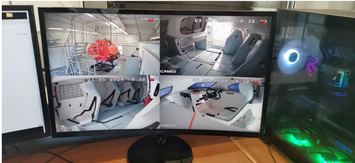
Video surveillance system control
